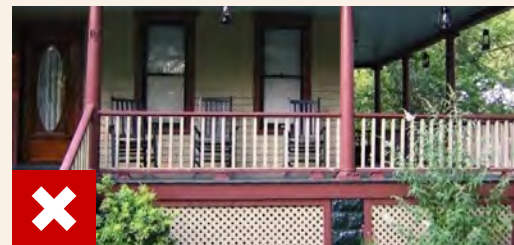
Handrail Height Too Tall
