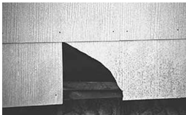
Figure 8.5: Asbestos-cement products most commonly deteriorate by cracking and chipping. These kinds of deterioration are not typically feasible to repair, and therefore it is recommended that a non-asbestos fiber cement piece be used as a replacement (photo by author).
