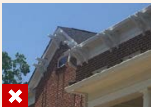
Inappropriate Eaves Returns and Eave Brackets
