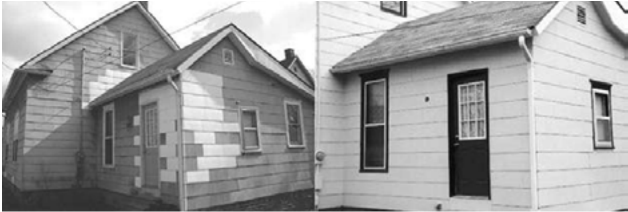
Figure 8.6: Replacement non-asbestos fiber-cement shingles in place, before being painted and after (photo by author).
