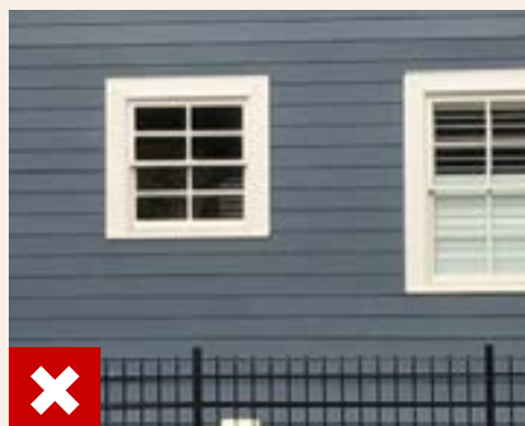
Inappropriate Window Configurations
