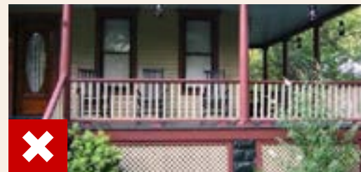
Handrail Height Too Tall
