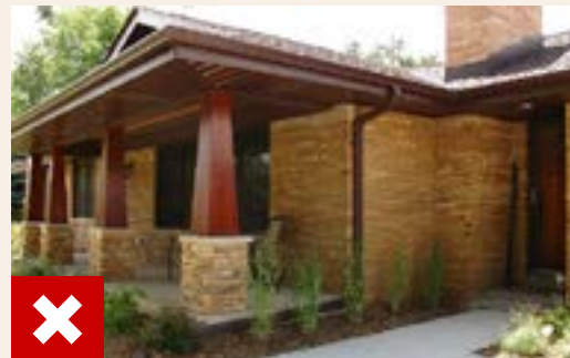
Inappropriate Porch Columns and Beam Details
