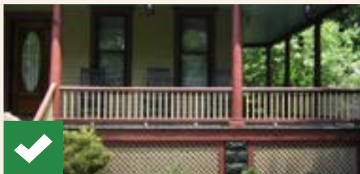
Historically Correct Handrail Height
