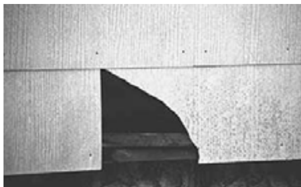
Figure 8.5: Asbestos-cement products most commonly deteriorate by cracking and chipping. These kinds of deterioration are not typically feasible to repair, and therefore it is recommended that a non-asbestos fiber cement piece be used as a replacement (photo by author).
