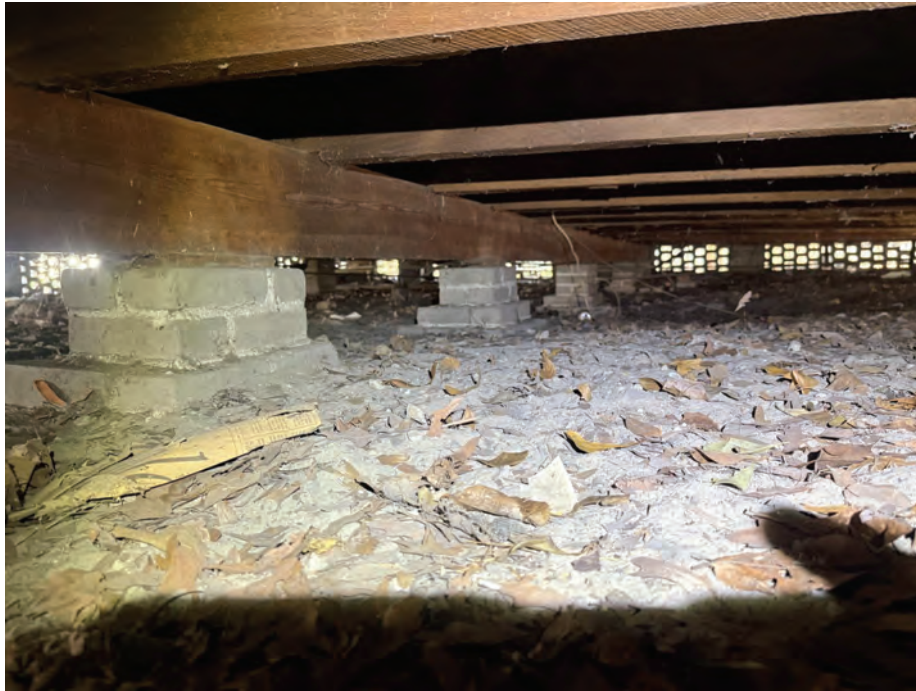
Figure 6: Crawlspace looking across the structure; concrete-block piers, soil floor with leaf litter, perimeter foundation vents at right. Photo taken by Chris Woods.
