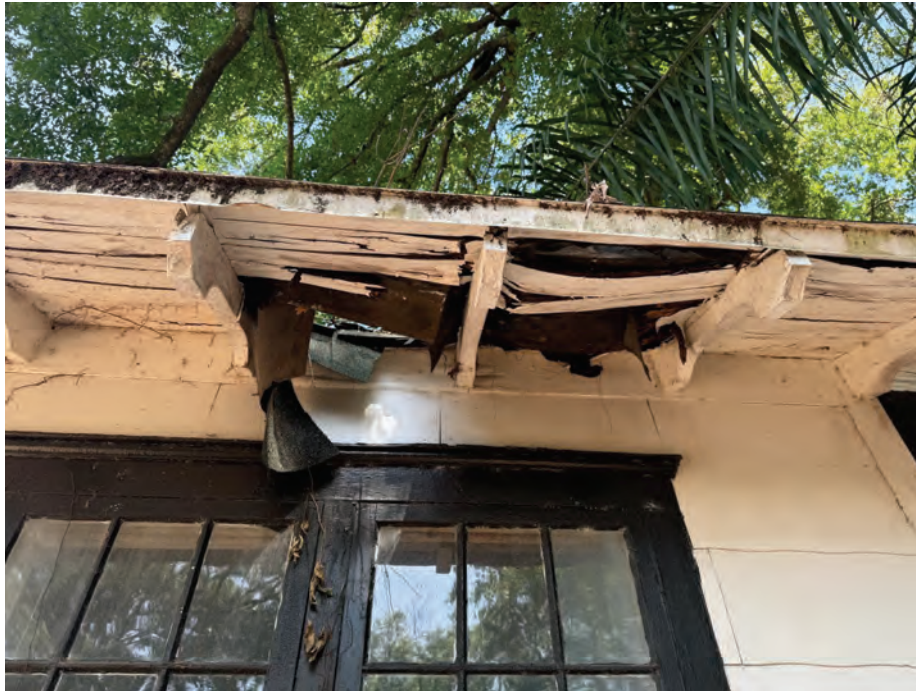
Figure 8: Eave above the windows; failed cornice and soffit between rafter tails, dropped roofing material, vegetation. Photo taken by Chris Woods.
