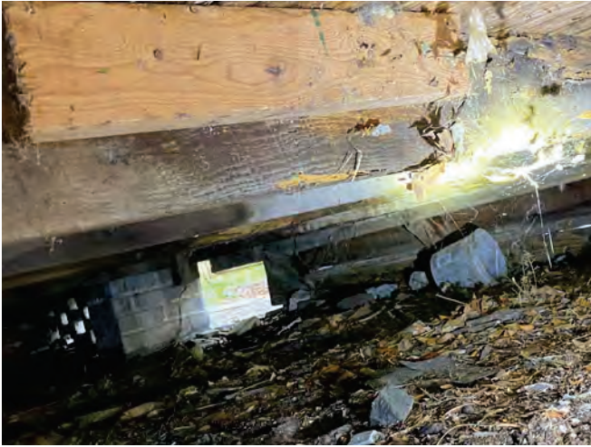
Floor Joist Damage & Prior Repair
