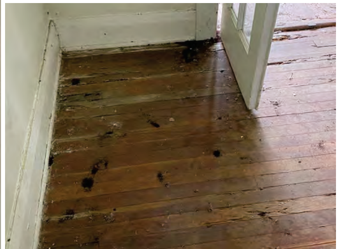
Bedroom Floor Damage & Termite Frass
