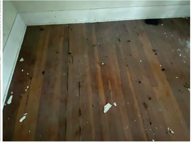
Termite Damage & Frass in NE Bedroom
