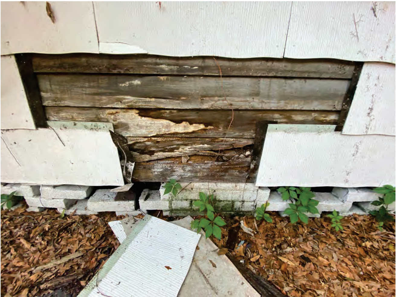
West Exterior Wall/Floor Interface in Dining Room
