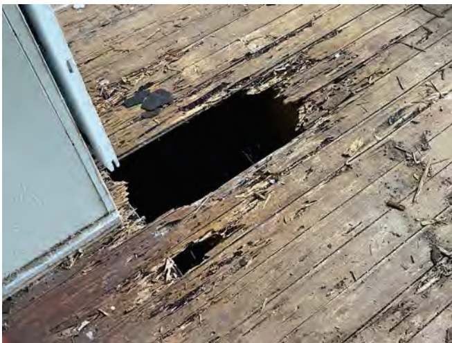
Termite Damage in East Sunroom Floor
