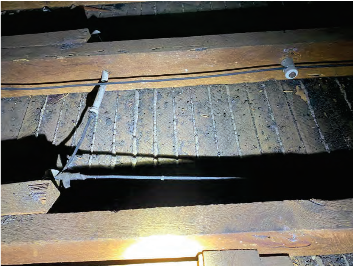
Knob-N-Tube Electrical Wiring in Attic
