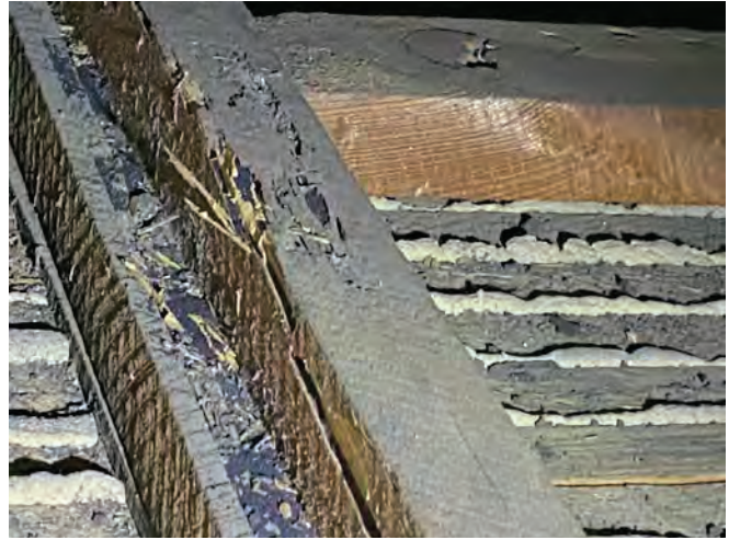
Termite Damage in Ceiling Framing
