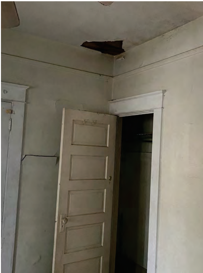
Bedroom Ceiling Damage
