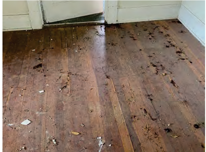
Termite Damage/Frass in Bedroom Floor
