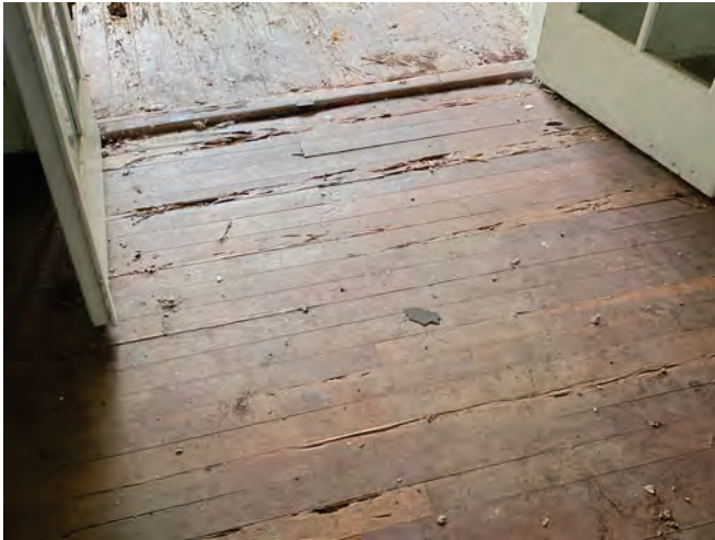
Termite Damage in Bedroom Floor
