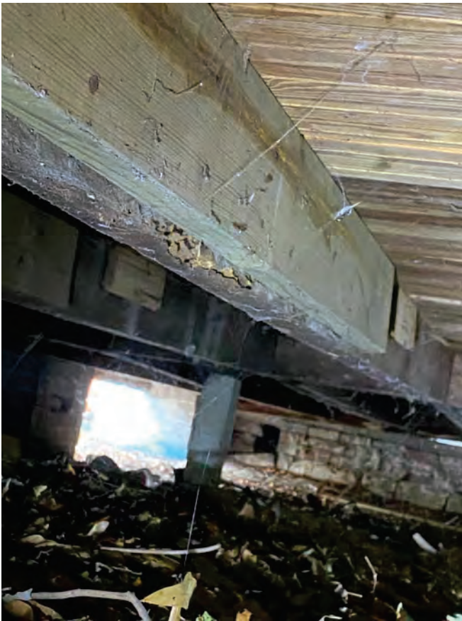
Damaged/Repaired Floor Joist
