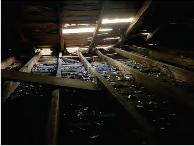
Roof/Ceiling Damage above Living Room
