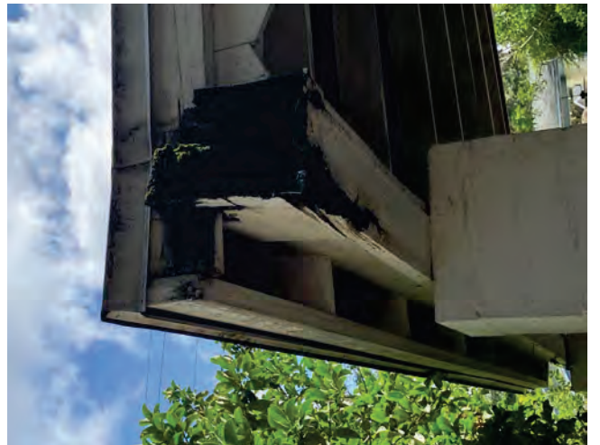
Southwest Corner of Carport Overhang
