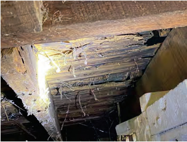
Damaged Floor Joist & Decking
