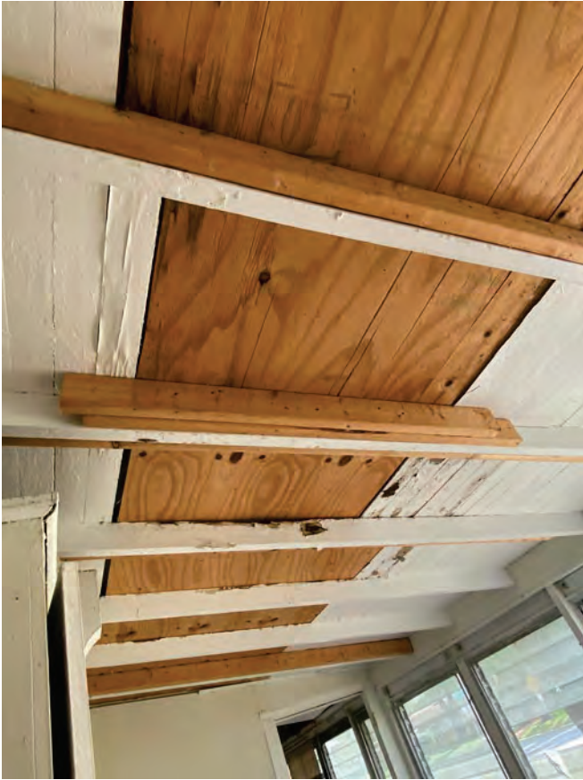
Prior Repairs to Sunroom Roof Framing
