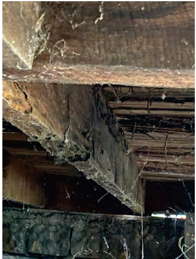
Damaged Floor Joist
