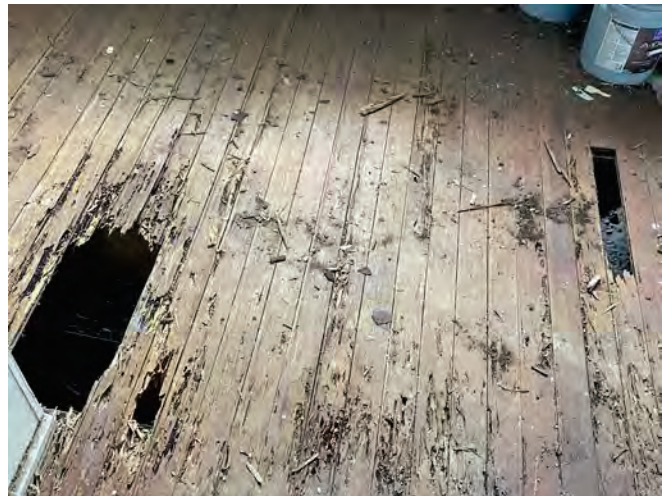
Termite Damage in East Sunroom Floor
