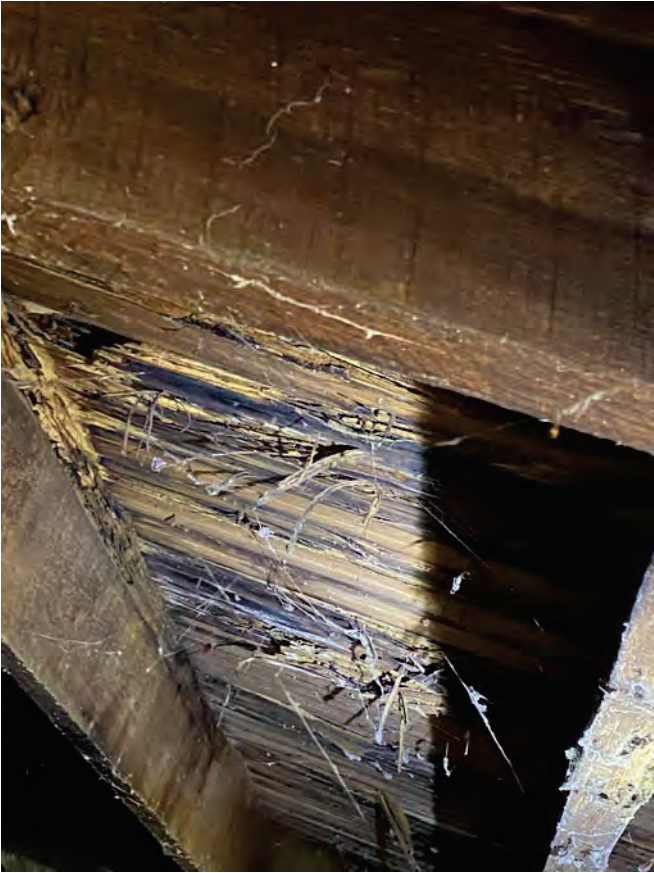
Damaged Floor Decking
