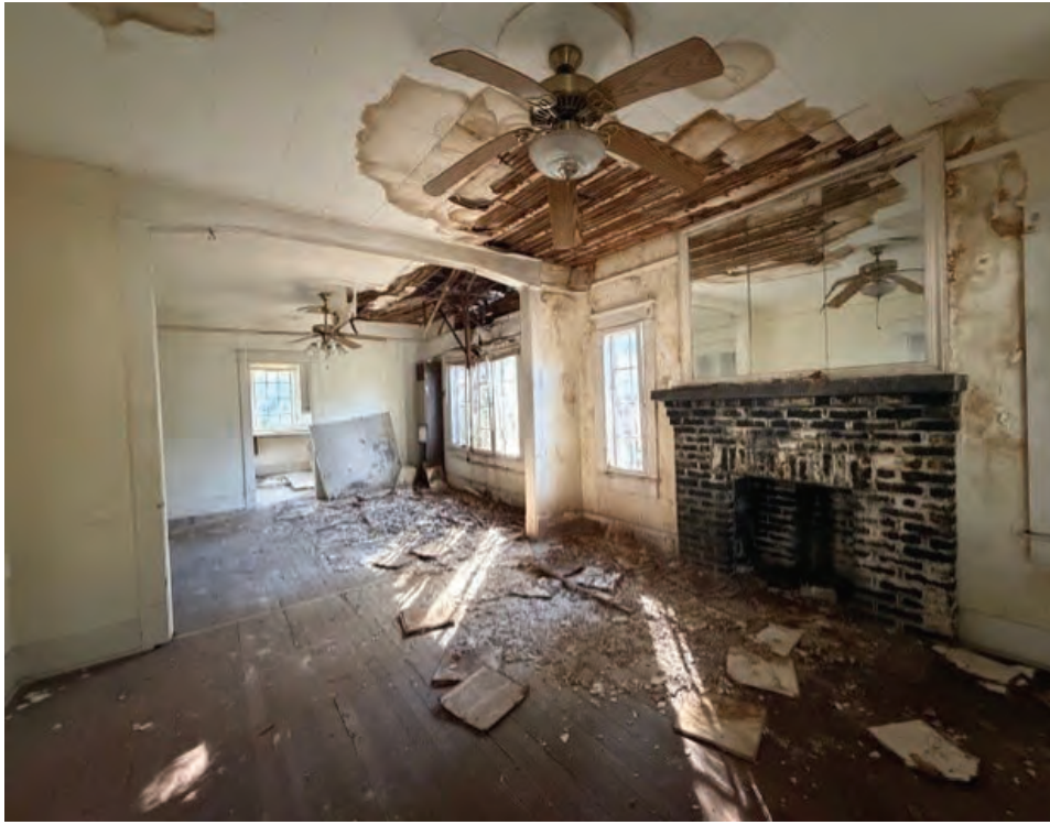
Figure 3: Interior wall in a principal room; window air-conditioner cut into wall between original wood windows, debris on floor, chimney mass at right. Photo taken by Chris Woods.
