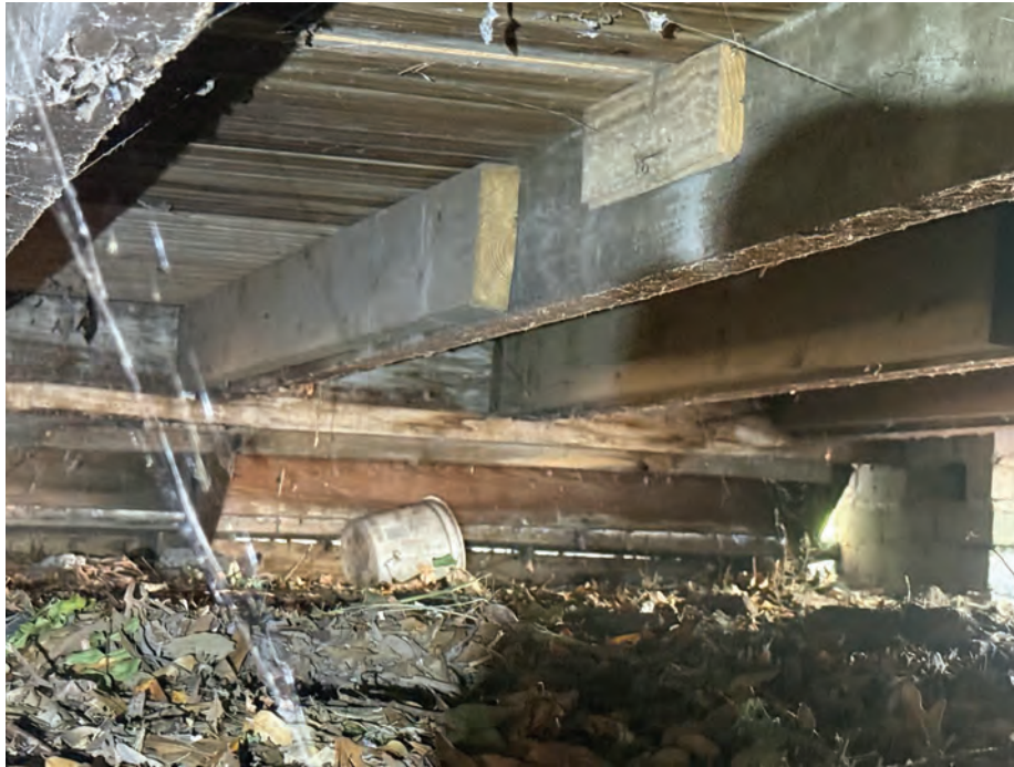
Figure 5: Floor framing from the crawlspace; original wood joists and beam with newer sister-board reinforcement (lighter, square-cut members). Photo taken by Chris Woods. Photo taken by Chris Woods.
