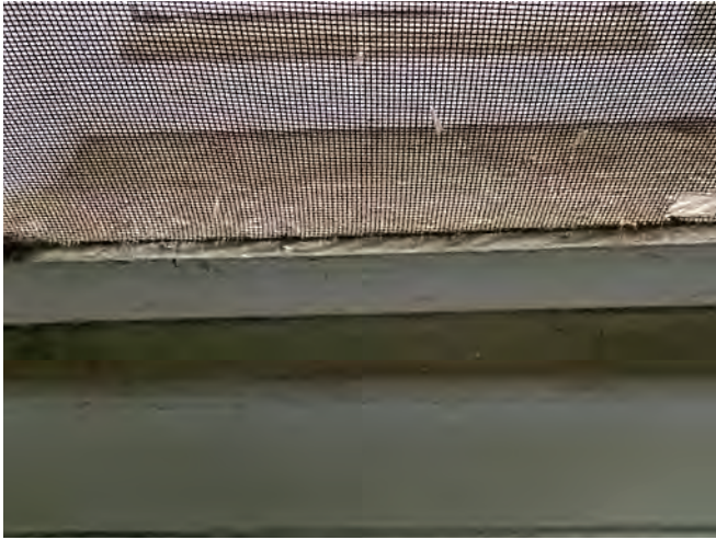
Drywood Termite Wings in NE Bedroom
