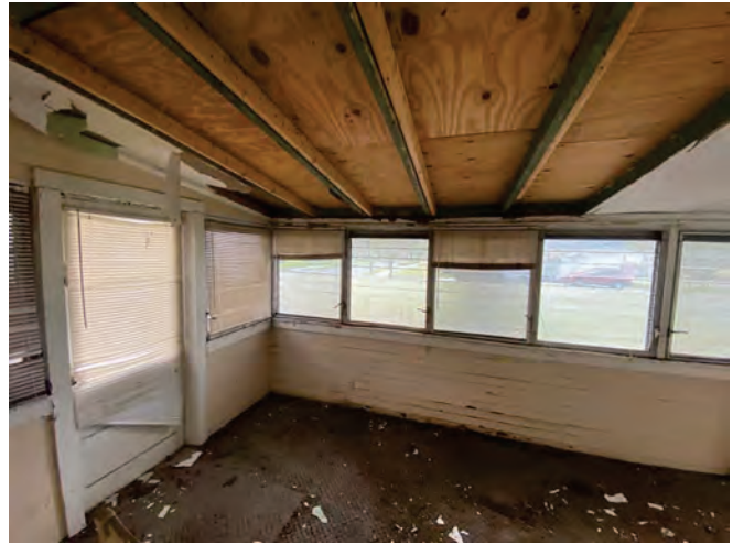
Prior Sunroom Roof Repairs & Floor Damage
