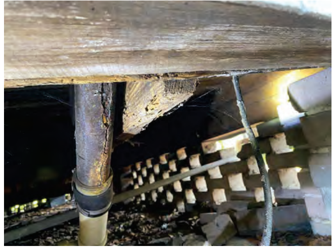
Floor Joist Damage & Rusted Out Plumbing
