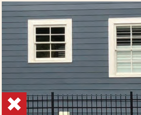
Inappropriate Window Configurations
