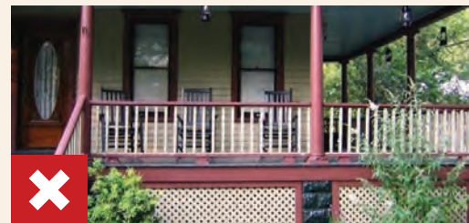
Handrail Height Too Tall
